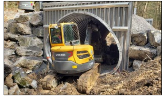
Photo 1: Placing larger material in a 15'w x 10'h pipe arch (squash pipe).
