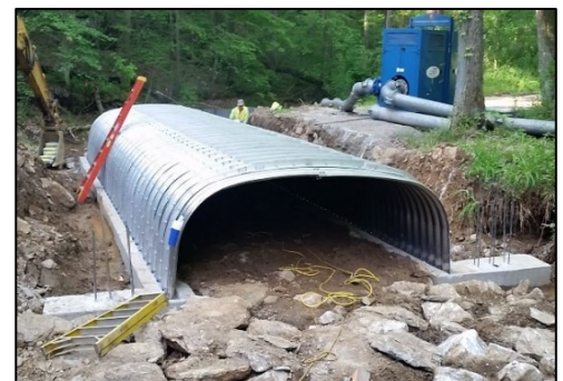
Bottomless arch pipe (York)
