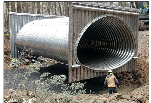
Installation of a 15' w x 10' h pipe arch that was assembled on site (CDGRS).
