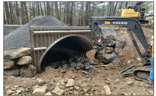
Photo 1: Placing grade control material in a 15'w x 10'h pipe arch (squash pipe).
