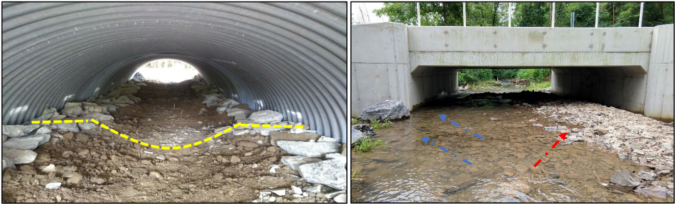
Figure 3: The photo on the left shows a properly constructed streambed with a low flow and bankfull channel, along with bank margins. The photo on the right shows a structure did not have a properly constructed channel and the resulting sediment deposition at the inlet forcing the flow to the side of the structure.
