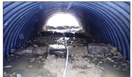
Photo 3: Grade control placed inside of a 15' wide arch pipe before placing final streambed.
