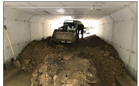
Photo 3: Placing fine material inside a bottomless concrete culvert with walk behind skid steer.
