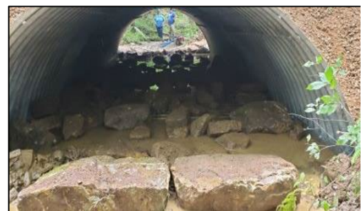
Photo 4: Large material placed in a 12'w x 6'h arch pipe before placing streambed.
