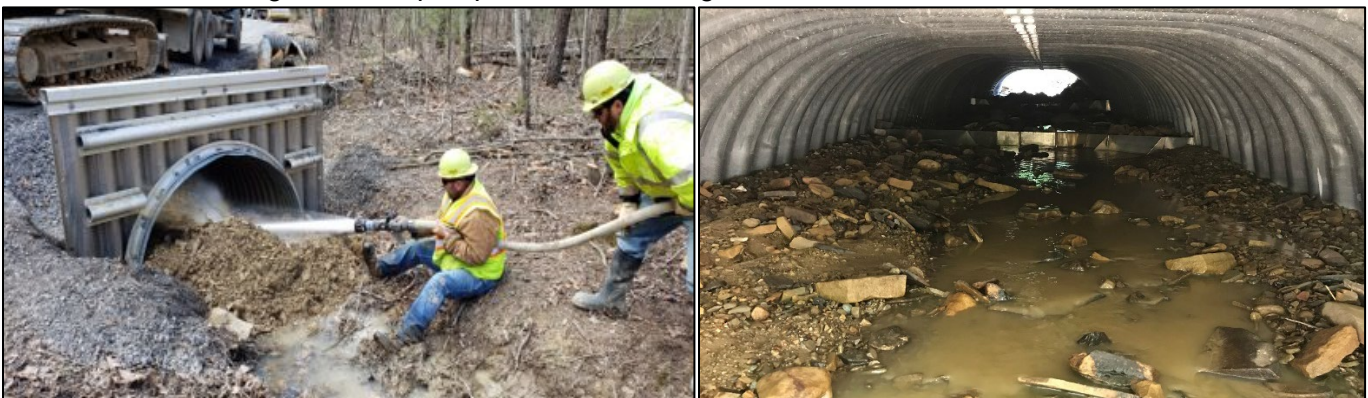
Figure 4: The photo on the left shows washing of fine material into a 6'w x 4'h pipe arch (squash pipe) using a fire truck. The photo on the right shows the washing process between tanker loads and view of a baffle grade control.
