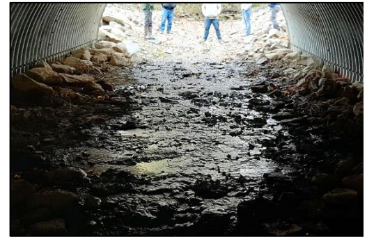
Bank margins established to create a low-flow channel and protect the structure from scour.
