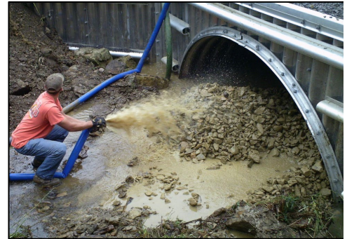
Washing fines into the streambed on a 12' w x 4' h pipe arch (Jefferson).
