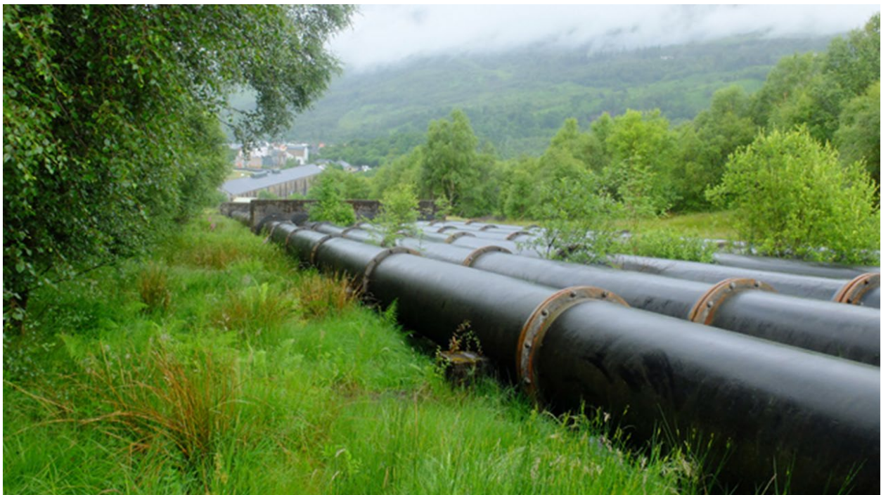
RPCO reviews and approves permit applications for pipeline construction among other project types. Copyright: John Allan and licensed for reuse under this Creative Commons License .
