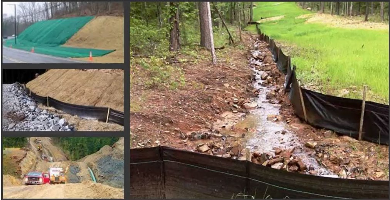
Examples of erosion and sediment control BMPs being installed to protect waters of the Commonwealth.
