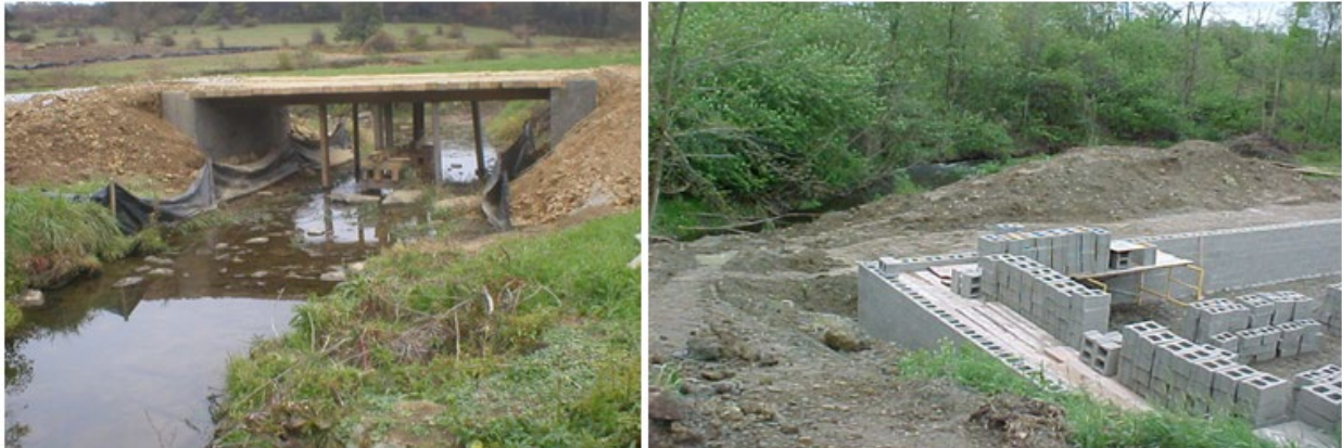
(Left): New construction or re-construction of a bridge over a stream channel. (Right): Structure being erected in the floodway of a stream. In both cases, these activities may require a permit under Chapter 105 regulations. Credit (both): PA DEP
