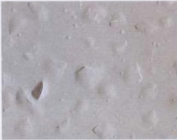
5. Blisters — Osmotics Small blisters — gel coat; large — laminate
